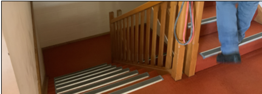
Figure J - Internal Stair Balustrades do not Achieve Height Requirement of 865mm.
