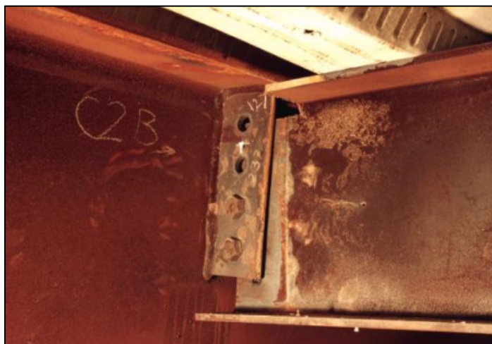
Figure 29 - Cardington Fire Test - British Test 2 - Failure of Steel Connections.
