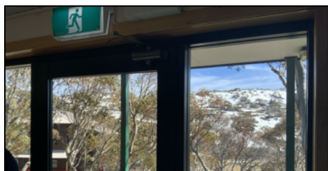
Figure N - Primary Entrance to have "OPEN INWARDS" Signage Installed.
