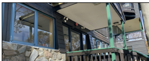
Figure O - Existing Fire Alarm System to be Upgraded to Comply with AS 1670.1-2018.
