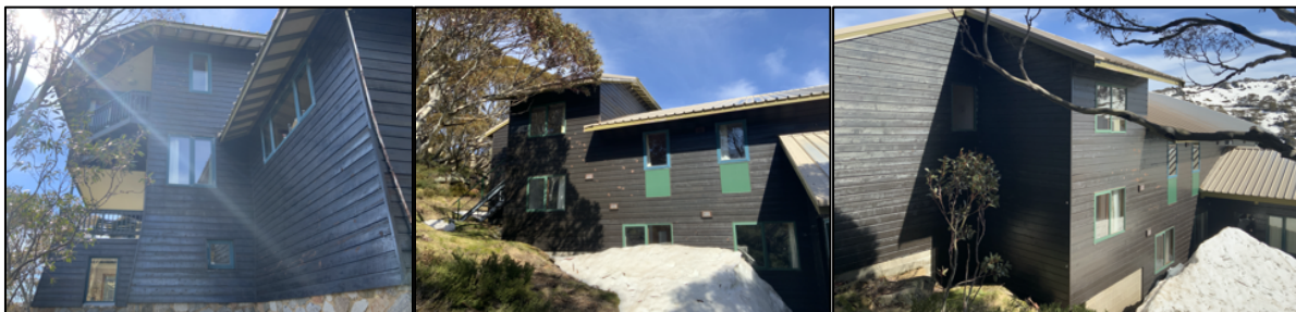
Figure 25 - Existing External Walls Consist of Combustible Elements.
