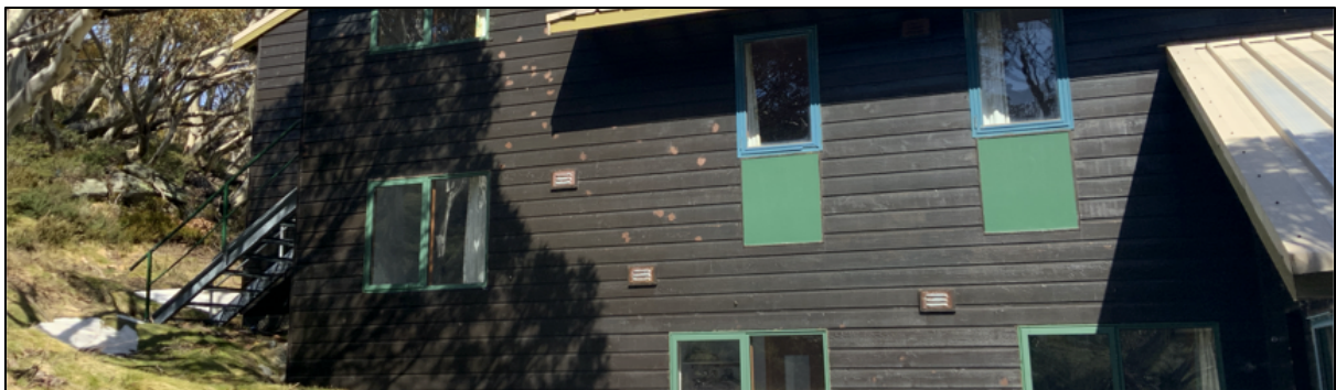
Figure 26 - Non-compliant Vertical Separation of Openings in External Walls.
