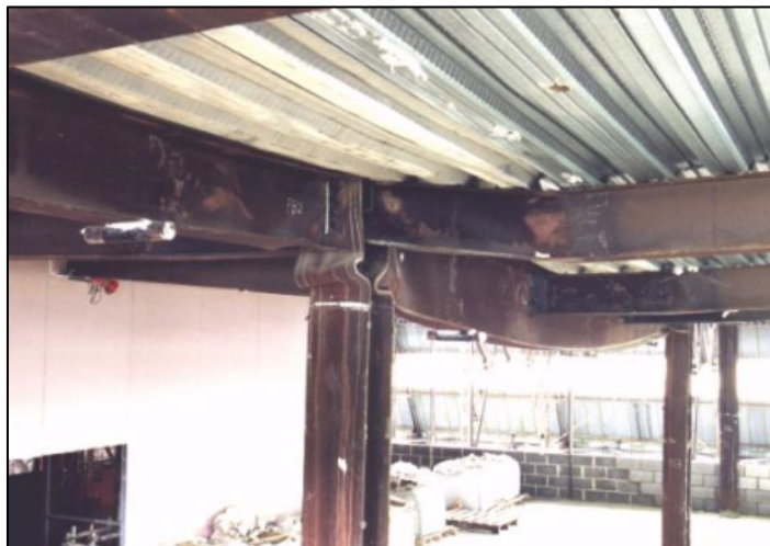
Figure 28 - Cardington Fire Test - British Steel Test 2 - Buckling of Unprotected Column.
